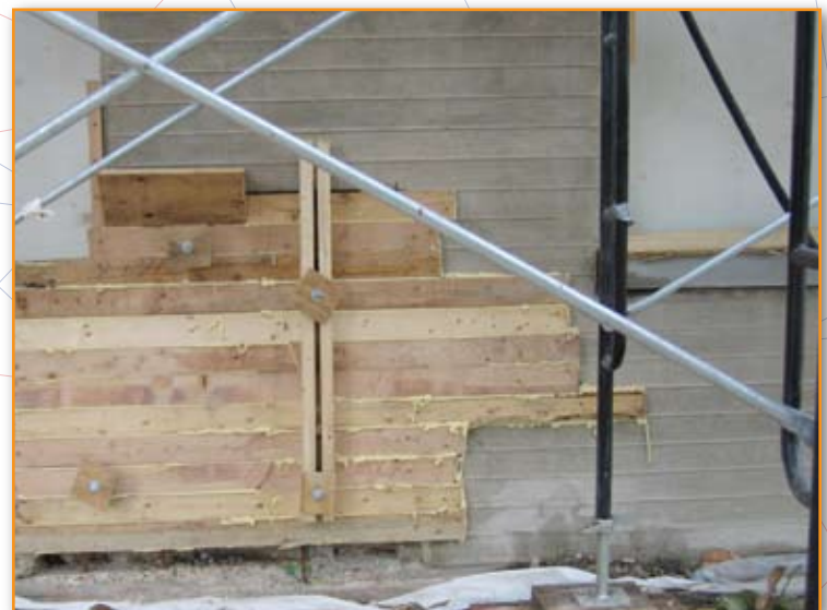
Figure 5: Formwork in place constructed to match original formboard finish on the existing walls.
