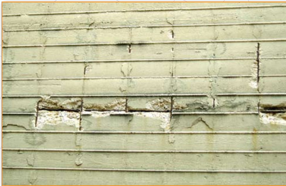
Figure 1: Typical lightwell wall damage showing spalling and exposed rusting reinforcing bars.
