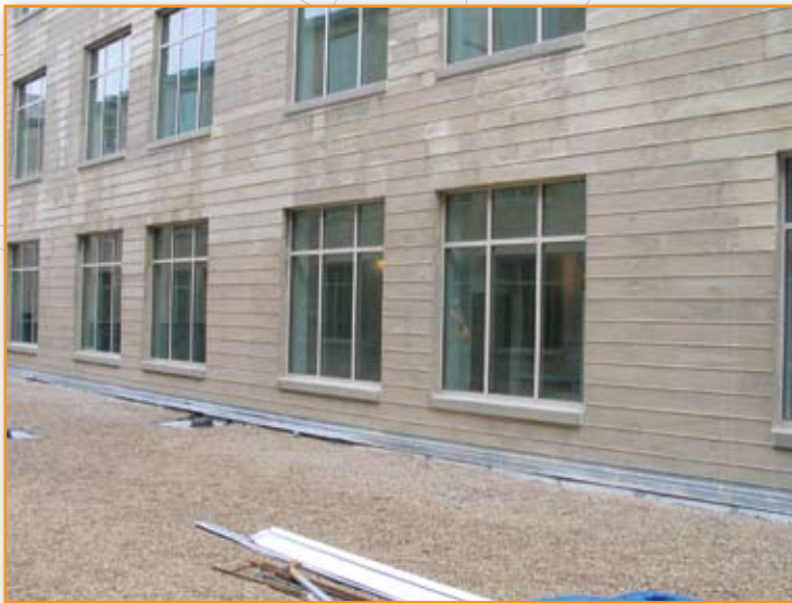
Figure 6: Portion of wall completed prior to application of silane and potassium silicate coating.
