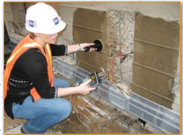
Figure 8: Corrosion rate monitoring of corrosion activity in unrepaired portion of wall adjacent to exposed corrosion damage.
