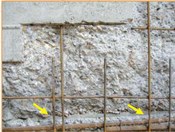
Figure 4: Close view of corrosion damaged reinforcing bars taken after completion of jackhammer demolition. Note the severe loss of cross section at the bottom of the vertical bars in the photo.
